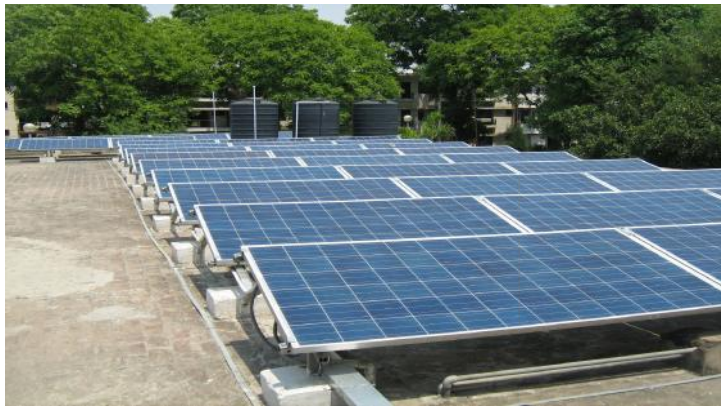
300 kwp CREST, Chandigarh(UT)
