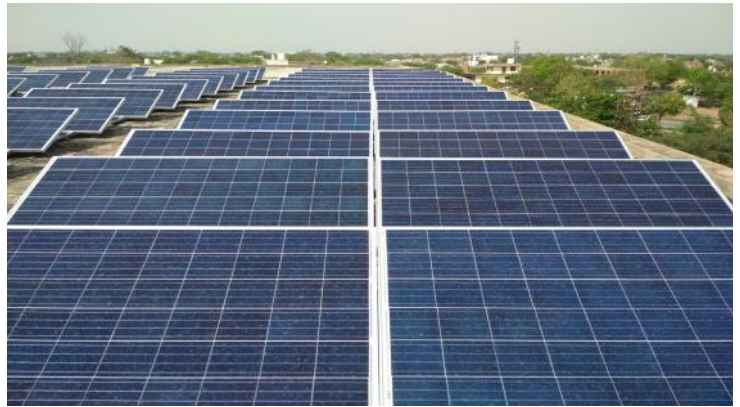
100 Kwp CEL, Indian Railways
