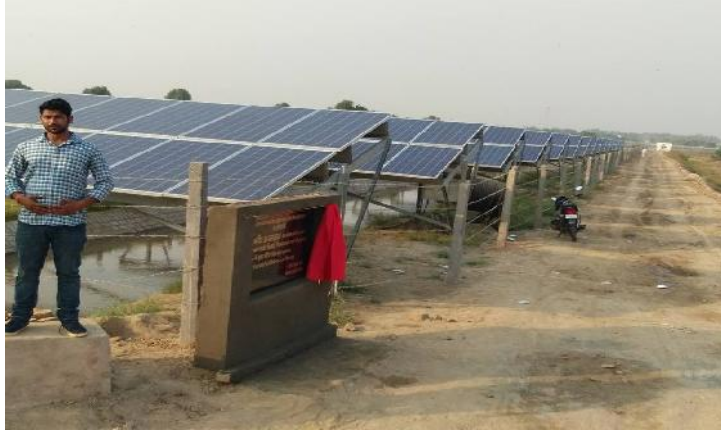
2 Mw [Utility Scale] Canal Based, Hanumangarh, Rajasthan
