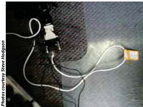
This extension lead has been tagged at each end, with different appliance numbers. Paid by the tag, perhaps?
