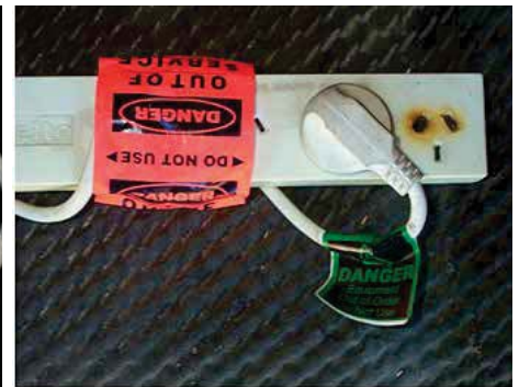
Don't plug heaters into power boards. A fire can result.
