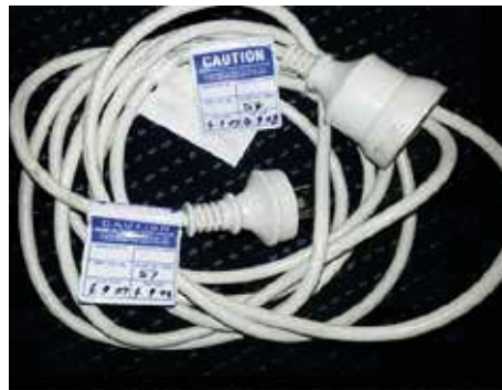
An "electrically qualified" person tagged this data lead unnecessarily.
